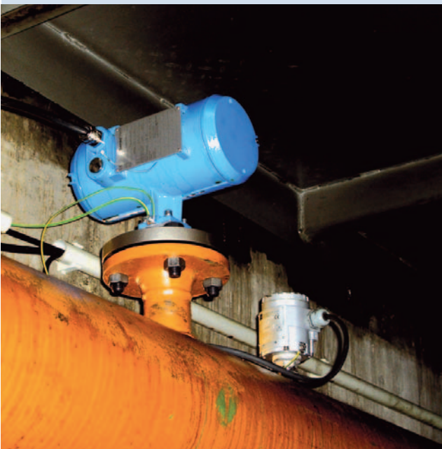
Figure 2. LiquiSonic sensor installed on the feeding line of a plant unit
